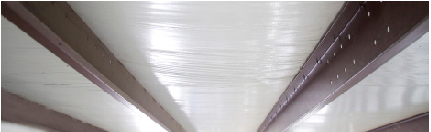
Interior view of the Dispense-R System
